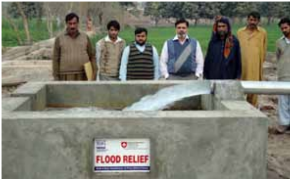
Water tube well installed by Nestlé and SDC for irrigation as part of flood relief activity
